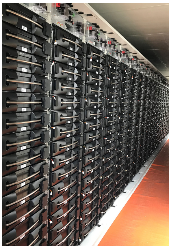
MPower is currently delivering a 5.6 MWh battery energy storage system for the Cook Islands incorporating lithium ion technology
